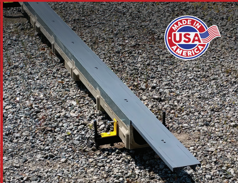
One 10' alignment frame supporting 3 channel sections and a catch-basin.
